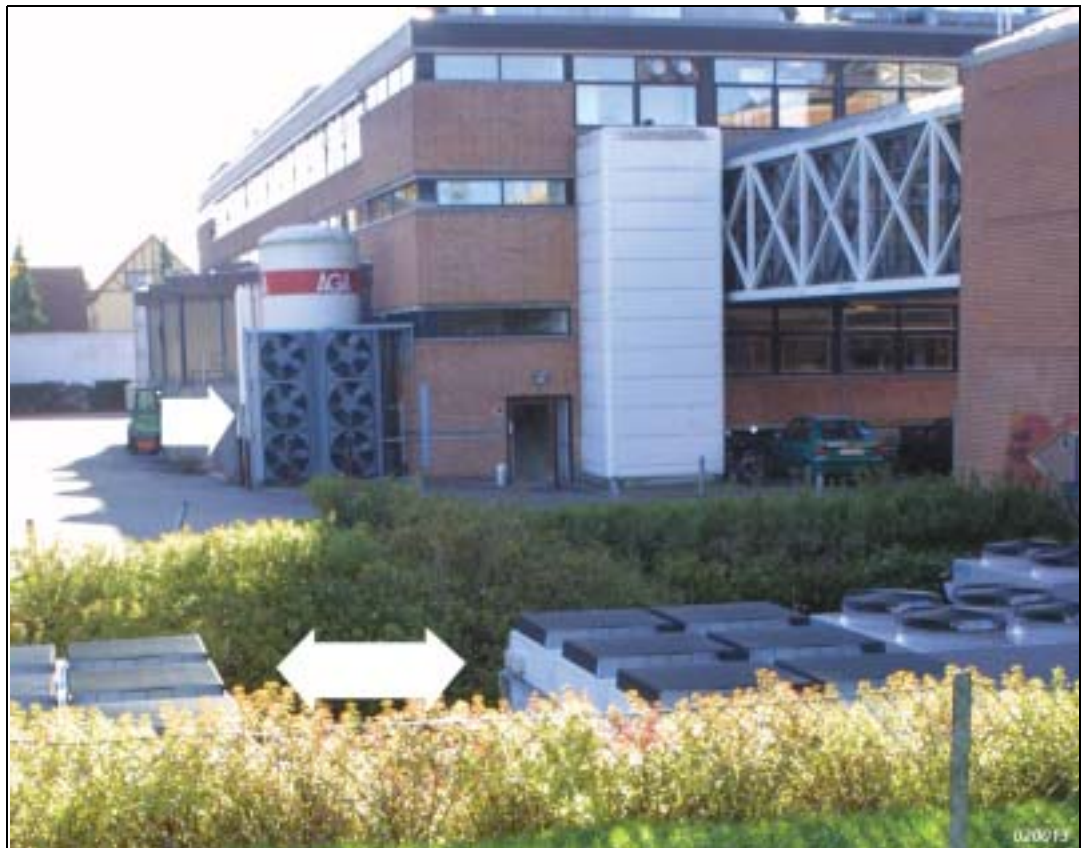
Fig. 1 Chemical plant with horizontal (close to fence) and vertical (on building) arrays of cooling fans
