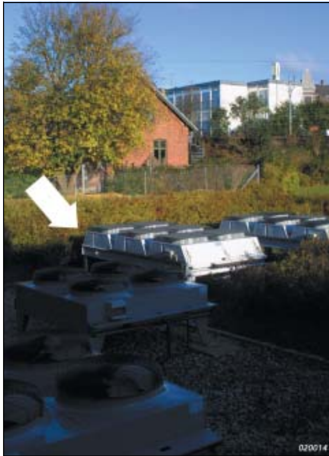
Fig. 2 Cooling fans located close to the fence of neighbouring dwellings
